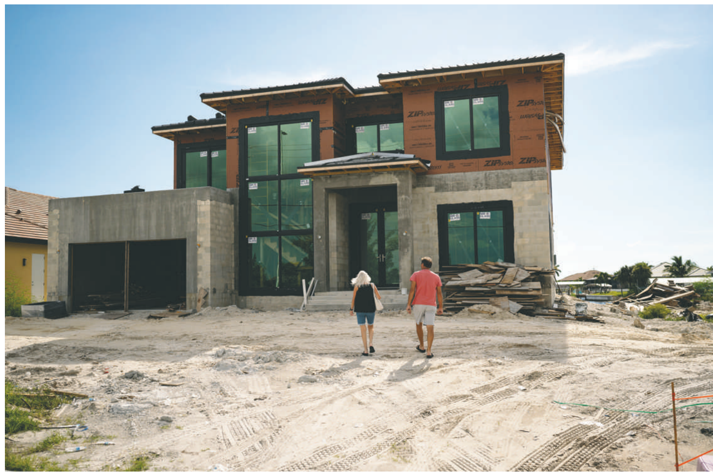
A residence under construction in July in Cape Coral, Fla., a canal-filled city vulnerable to sea-level rise and storm surge.
