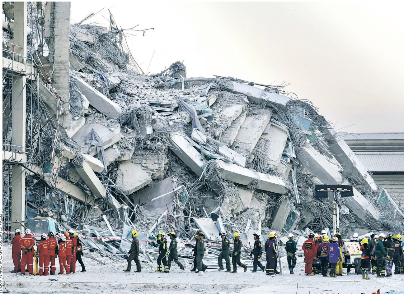
DESTRUCTION: Rescuers worked Friday at the site of a high-rise under construction that collapsed in Bangkok when a series of tremors struck Myanmar, where scores of people were killed. For video of the collapse, scan the code with the article on A8 .
