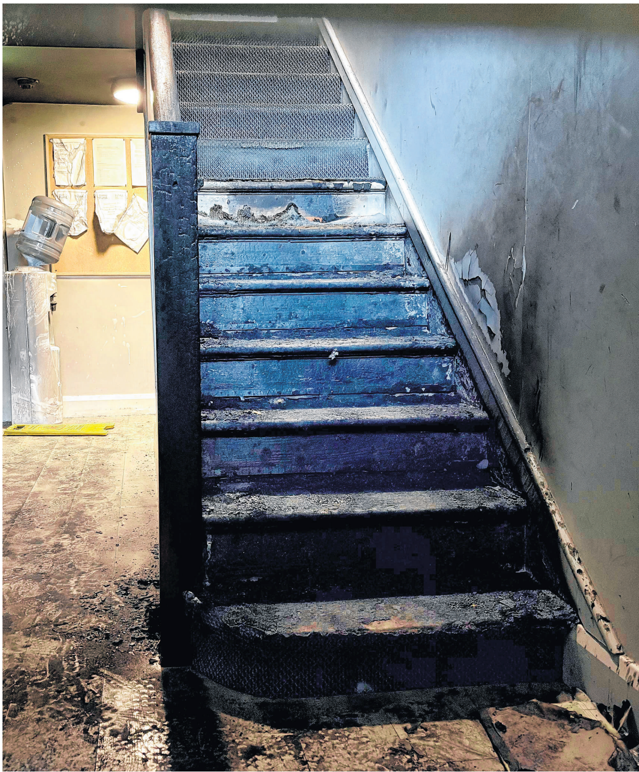
■ Damage to a staircase at an IPAS centre in Drogheda, Co Louth, caused by a suspected arson attack on Friday night.
