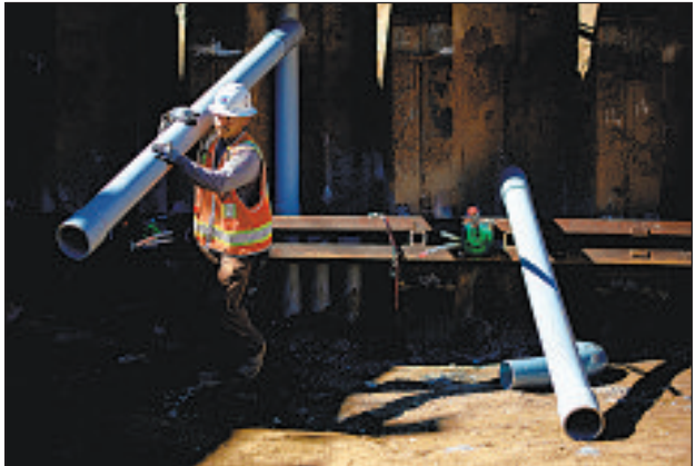
NEW FACILITIES at a DWP plant in Van Nuys will be able to purify enough water for 500,000 people.
