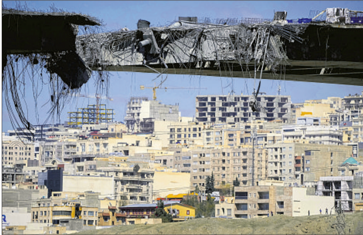
THE B1 BRIDGE, Iran's largest, was struck by U.S.-Israeli strikes late Thursday in Karaj, west of Tehran. VAHID SALEMI Associated Press
